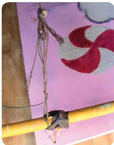
Avoid rigging like this! For tips on maintaining a safe rigging system, see Tom Young's feature on page 20.
