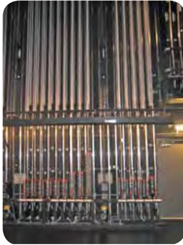
A counterweight rigging system in good working order.
